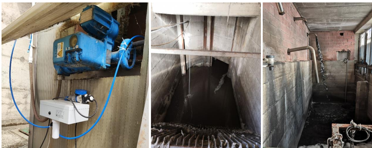
Figure 1. The WT1 installed outside the arrival tank (on the left), the inlet section of arrival tank (in the middle) and the second section of the arrival tank (on the right) with sludge recirculation active.
