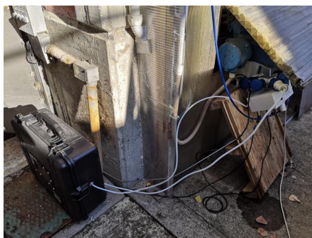
Figure 2. The airtight suitcase placed nearby the WT1 outside of the arrival tank.
