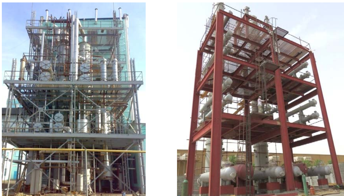
Figure 9: Cyclic distillation column as part of a plant producing ethanol in the food industry (left), and two cyclic distillation dividing-wall columns installed for fractionation of kerosene (right).
