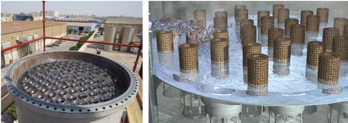
Figure 6: Top view of an installed cyclic distillation tray column with a diameter of 1.7 m (left), and visualization of cyclic distillation trays suited with solid catalysts for catalytic distillation applications (right)
